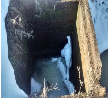
Figure 7. Shaft of ME with leakage from shut-off valve without manipulation device
