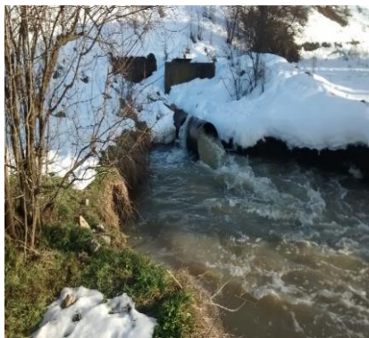
Figure 9. Attack on the metal pipe of the main exhaust
