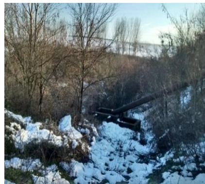
Figure 10. Mounted siphon for main exhauster
