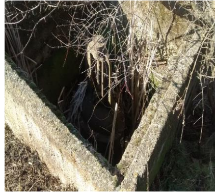
Figure 8. Shaft of clogged main exhauster with shut-off valve
