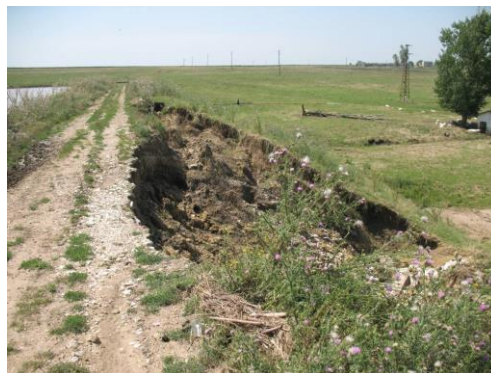
Figure 6. Damage crest area after overflow [19]
